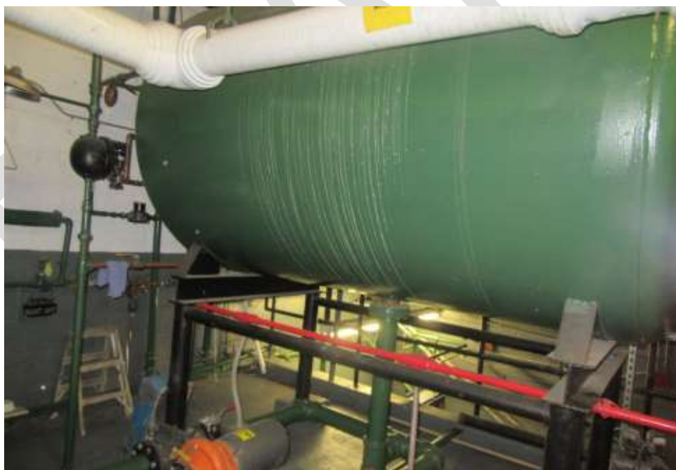
Boiler Feed Unit
