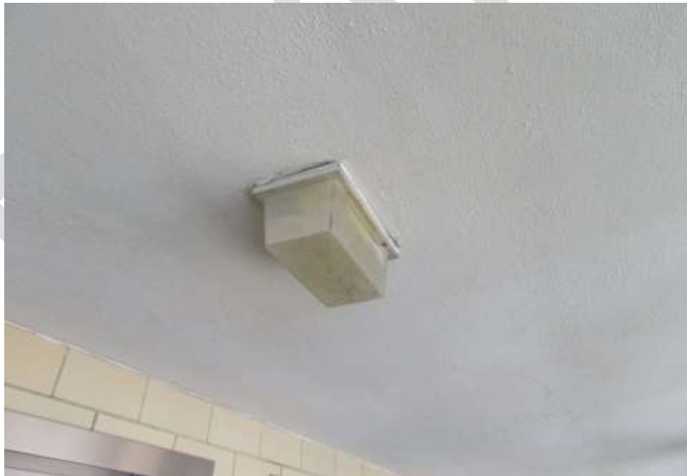
Typical Exterior Hallway Lighting Fixture
