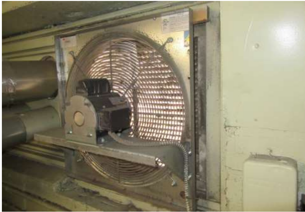
Typical Laundry Room Exhaust Fan
