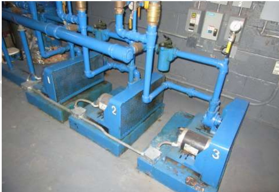
Fuel Oil Pumps
