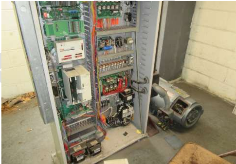
Typical Elevator Control Panel and AC Generator
