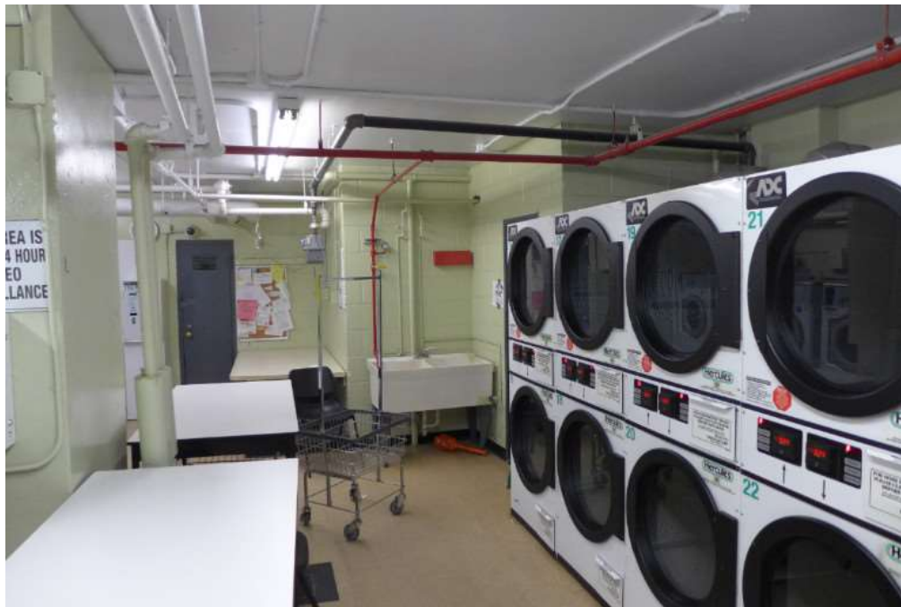
Typical laundry room
