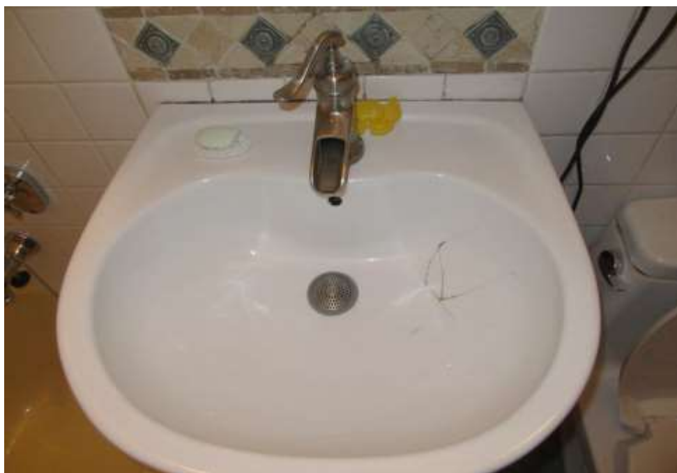
Typical Apartment Washing Sink
