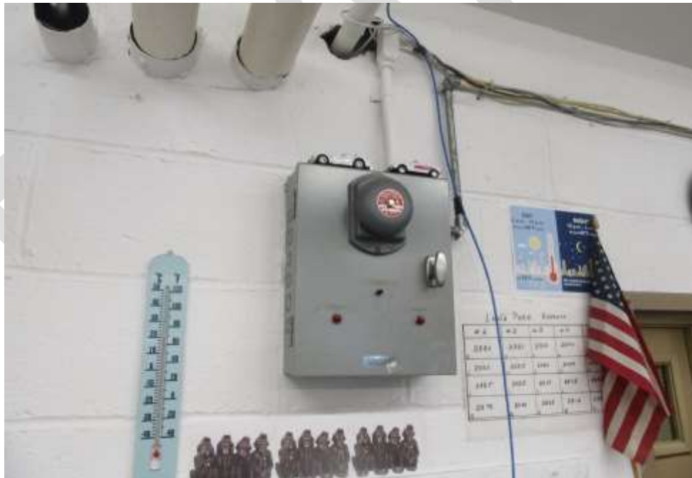
Water Tank Alarm Panel
