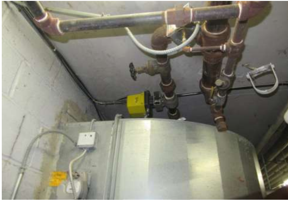
Typical Elevator Shaft Unit Heater Motorized Valve
