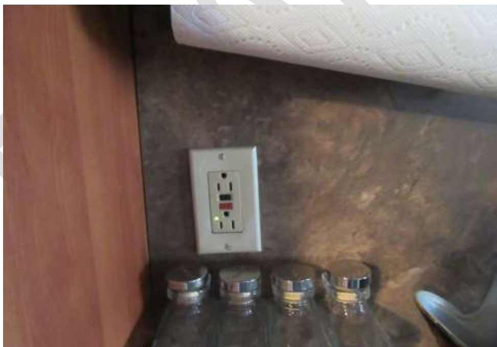
Typical Apartment GFIC Outlet in Kitchen
