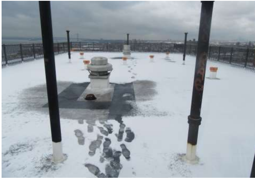
Typical Roof Exhaust Fans
