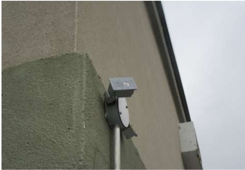
Typical Roof Lighting Fixture Day Light Sensor
