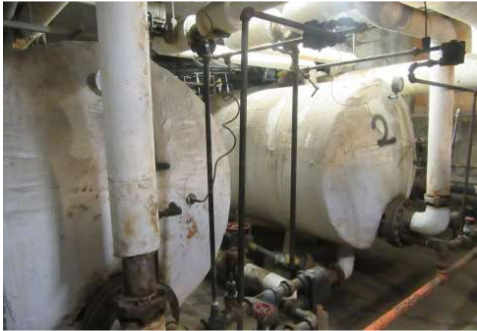
Typical DHW Storage Tanks
