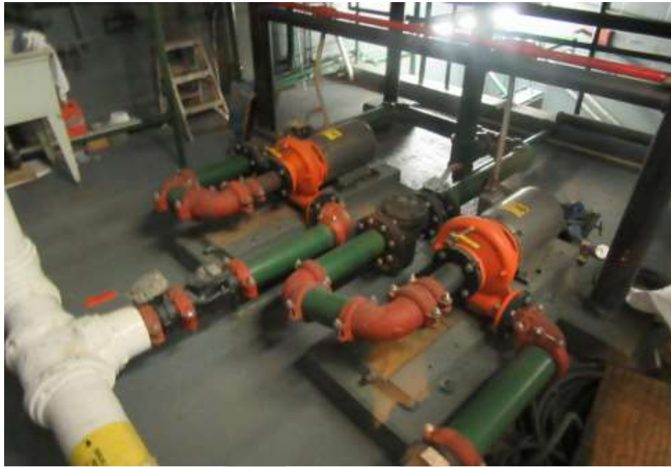
Boiler Feed Unit Pumps
