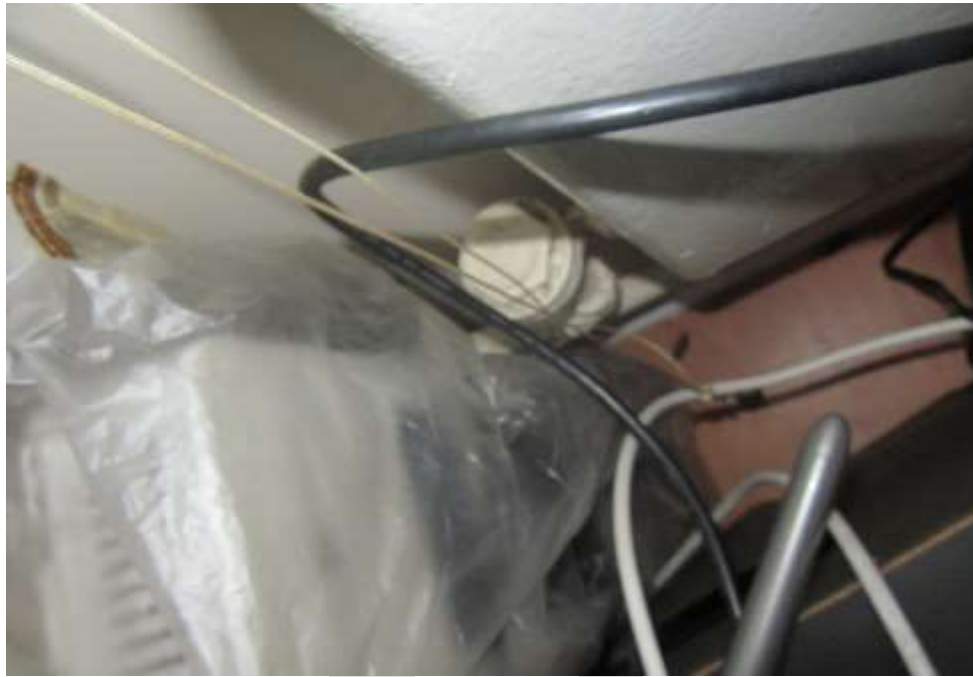
Typical Apartment Radiator Trap
