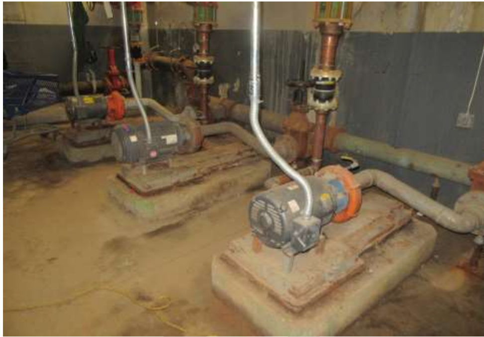
Building House Pumps
