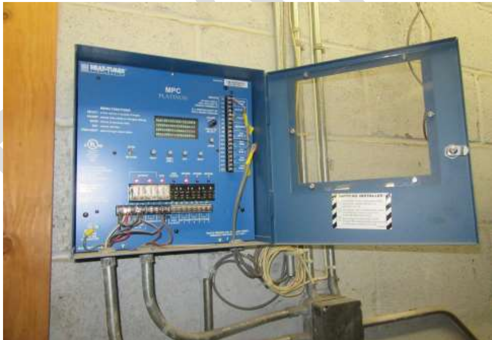
Typical Elevator Shaft Unit Heater Controller
