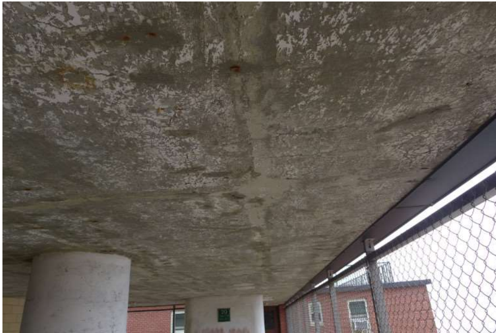
Underside of exterior walkway. Note the dark metal edging (on the right hand side) that conceals and holds up the broken concrete at the edges.
