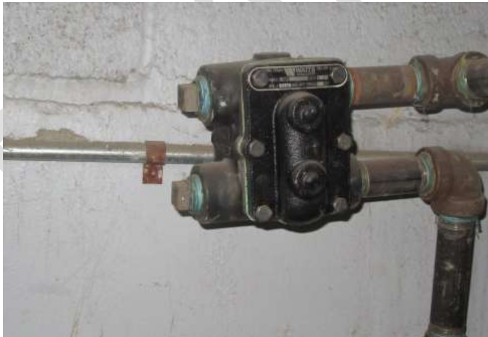
Typical Common Area F&T Trap
