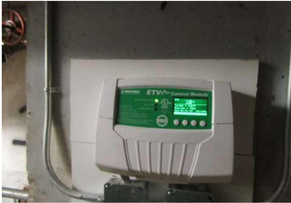
Typical DHW Motorized Mixing Valve Control Panel
