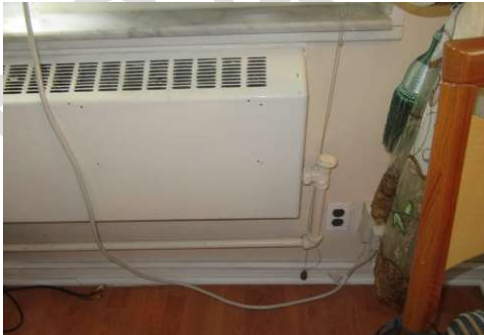
Typical Apartment Radiator Valve
