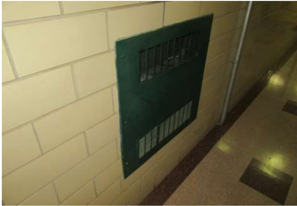
Typical Hallway Radiator
