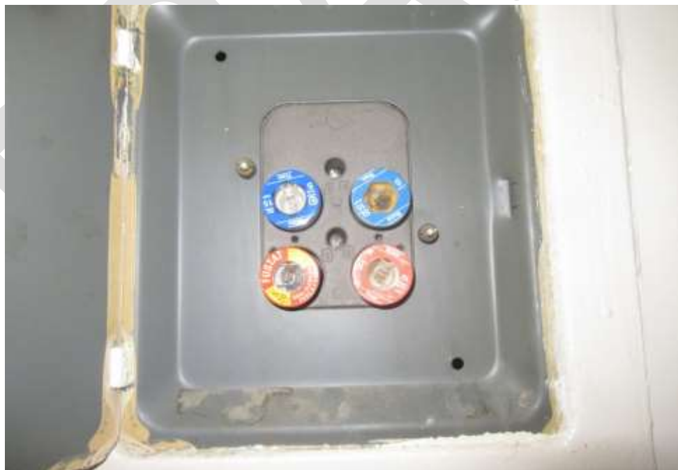
Typical Apartment Original Fused Panel
