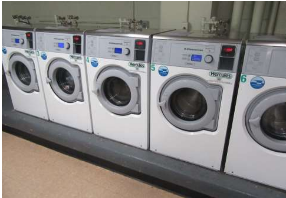
Typical Laundry Washers
