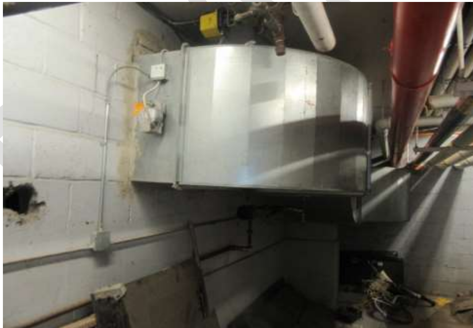
Typical Elevator Shaft Unit Heater
