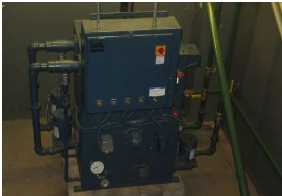
Typical Vacuum Pump Set
