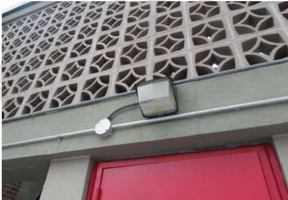
Typical Roof Lighting Fixture
