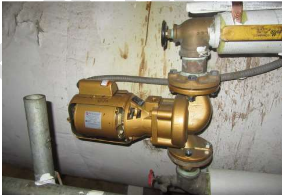
Typical DHW Circulation Pump
