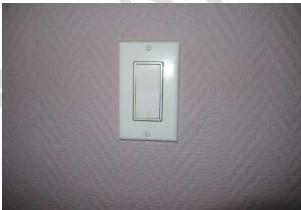
Typical Apartment Switch
