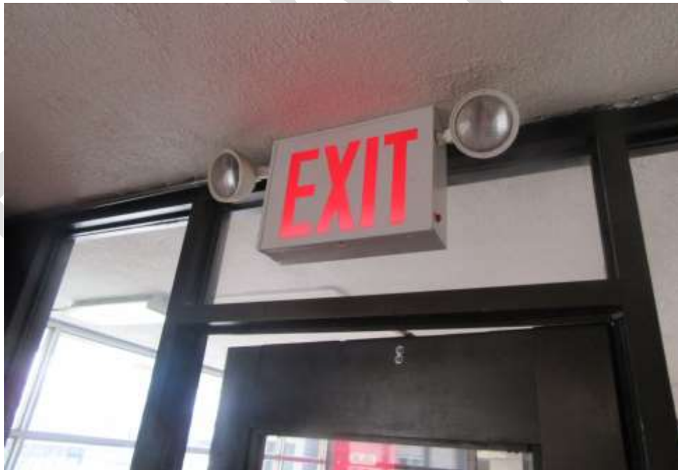
Typical Exit Sign with emergency Heads
