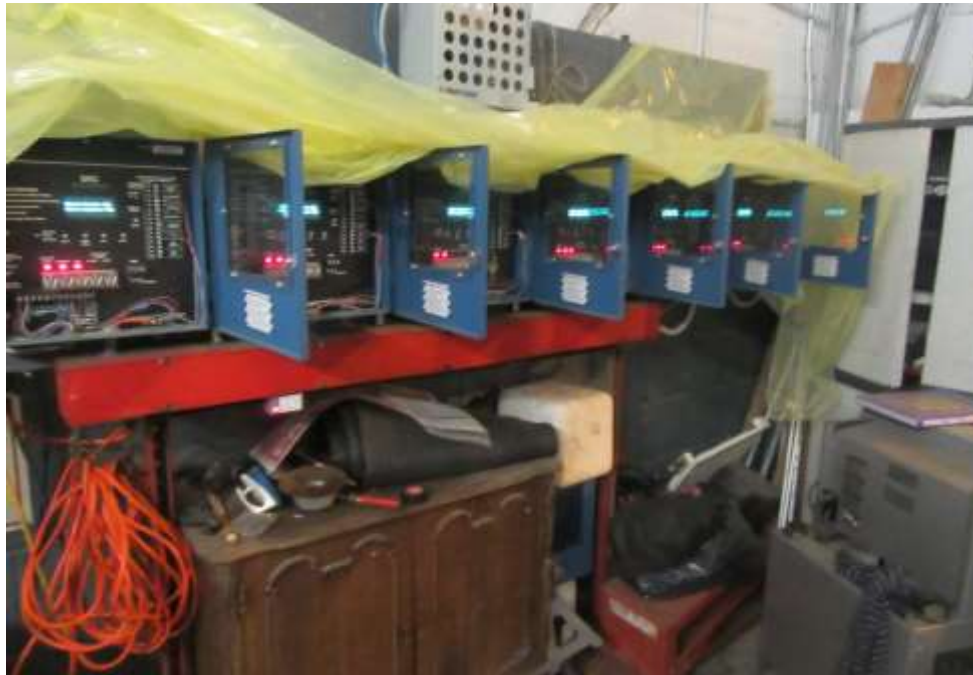
Heating Motorized Valves Control Panels
