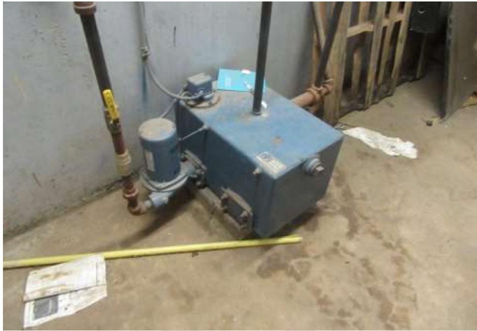
Typical Condensate Receiver
